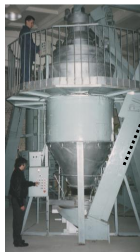
The gas generator and furnace in one unit
